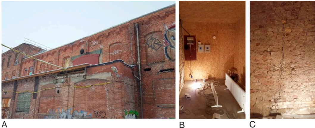
Figure 3. A) Industrial building from 1896 south of Gothenburg to be insulated on the interior with VIP, B) The test room inside the industrial building, C) Sensors in the external brick wall. Photos: Pär Johansson.
