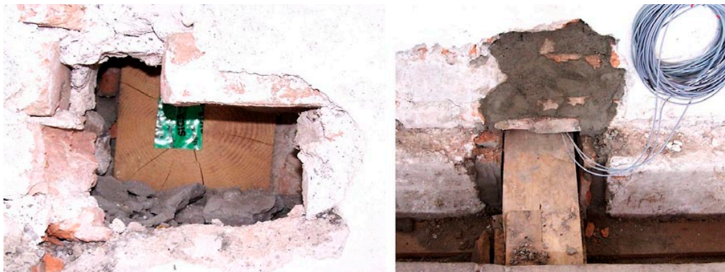
Figure 9. Variant N4/4b with fresh mortar in direct contact to the beam head (left) and. variant N5/3 with a lot of built in mortar (right). Photos: Fraunhofer Institute for Building Physics IBP.
