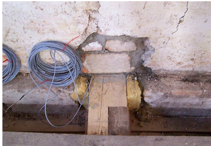
Figure 2. Variant 1 with common halving, mortar bed and insulation mounted around the beam head. Photo: Fraunhofer Institute for Building Physics IBP.
