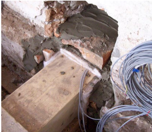
Figure 4. Variant 5 with common halving, aerogel mat around the beam head and as support. Photo: Fraunhofer Institute for Building Physics IBP.
