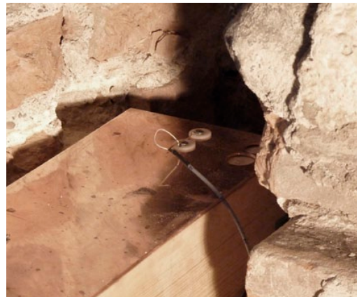
Figure 5. Variant 6 with a copper plate as an artificial thermal bridge. Photo: Fraunhofer Institute for Building Physics IBP.
