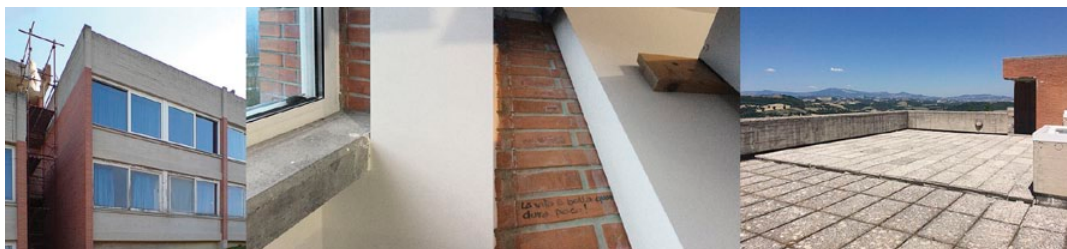
Figure 8. After the pilot site, from left to right: new window, “cold wall” insulation, slab cover.
